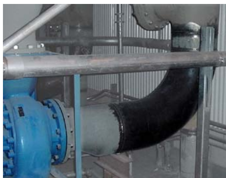
Vortab VEL installation at pump inlet
