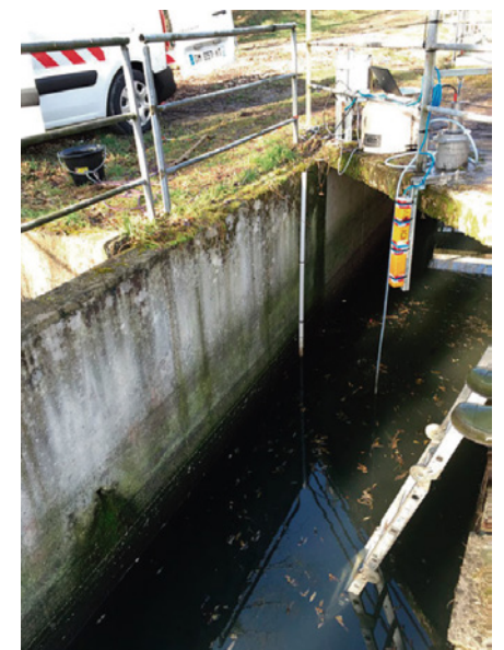
Municipal Rainwater Collector, France
