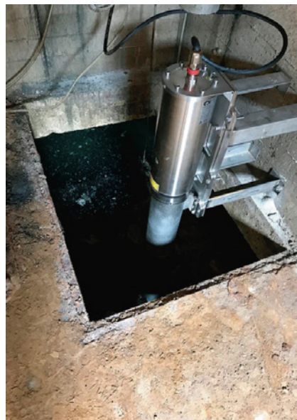
Fuel depot, water cistern, Norway
