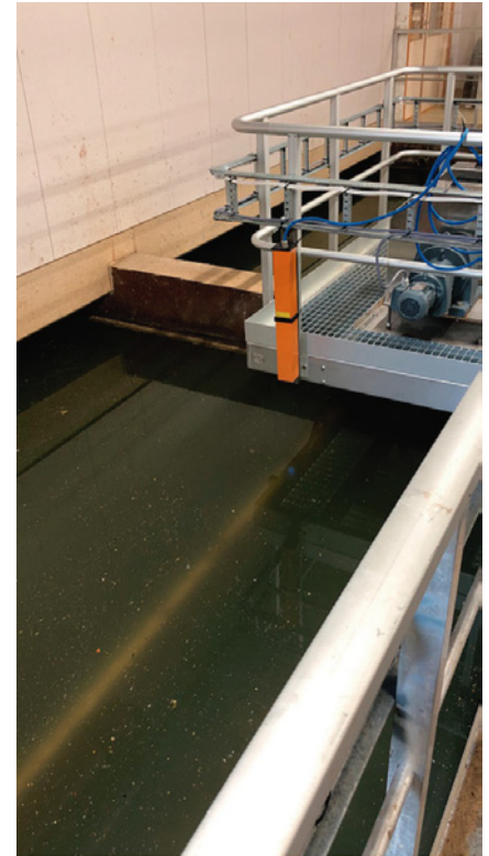
Waste Water Treatment Plant - Norway
