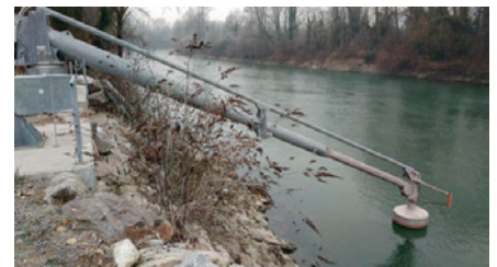
River Pumping Station, France
