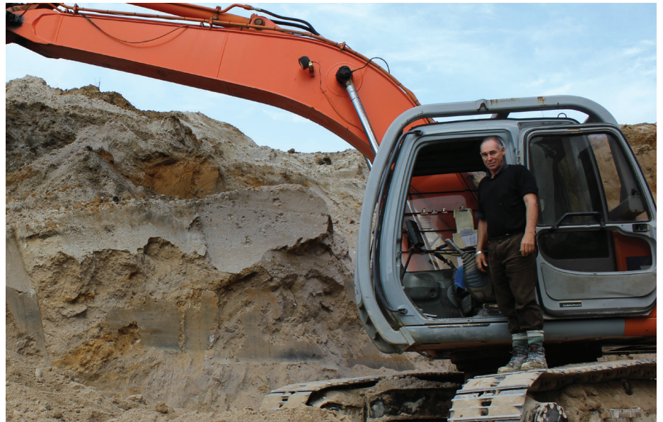
Richard is a happy man after installing the LOADRITE X-2350 on his excavators
