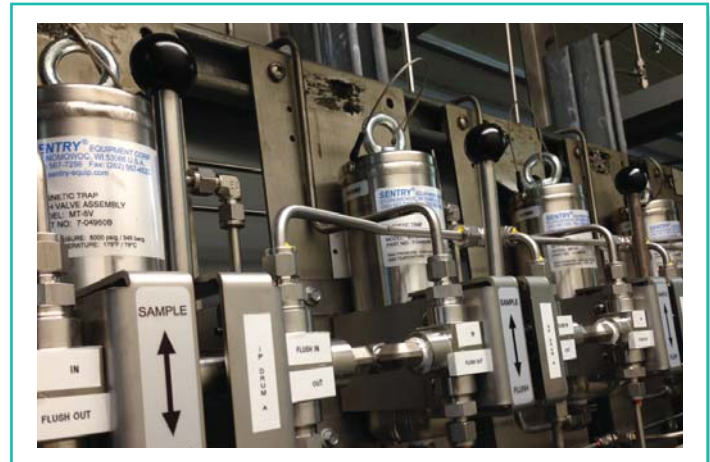
A 2x1 combined cycle power plant in the southeastern U.S. has experienced success with the Sentry MT Series magnetic trap. The installation – with magnetic traps for the HP drum and IP drum – is shown above.
