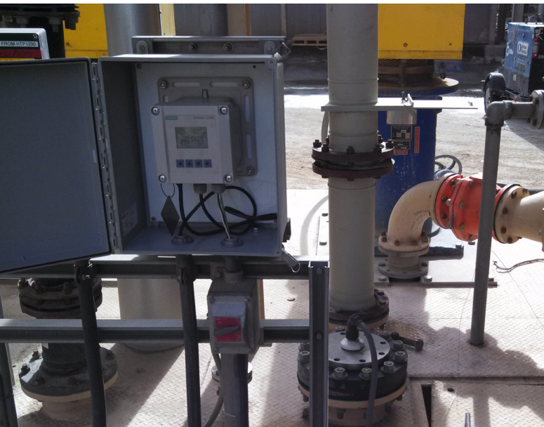
Commissioning the SITRANS LUT400 was very easy – with the controller’s Quick Start Wizard, the new level measurement system was up and running in record time.
